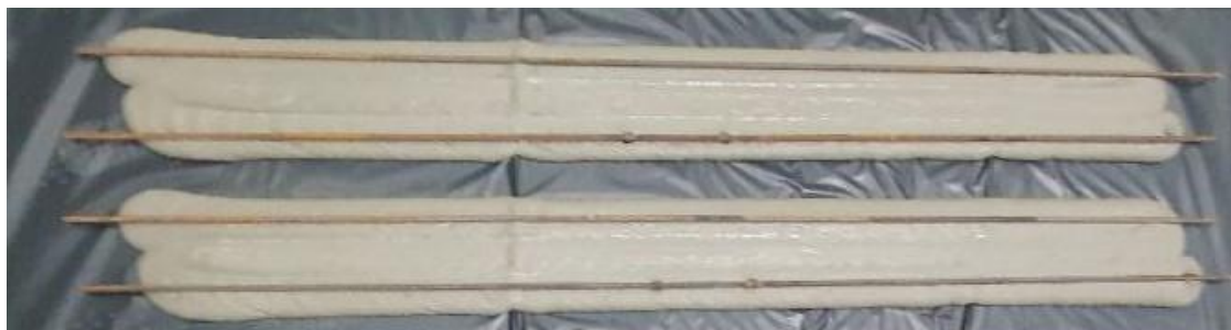
Fig. 3. Reinforcement with individual reinforcing bars along the first layer of the printer
